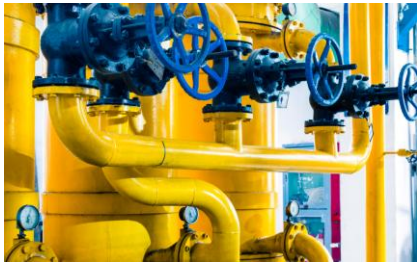
Gas-control equipment. Industry illustration.
